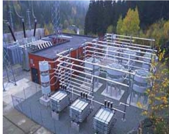
400 kV, 320 MVAR SVC Installation
