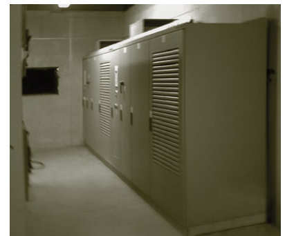
ACS 1000, controlling the cane mill
