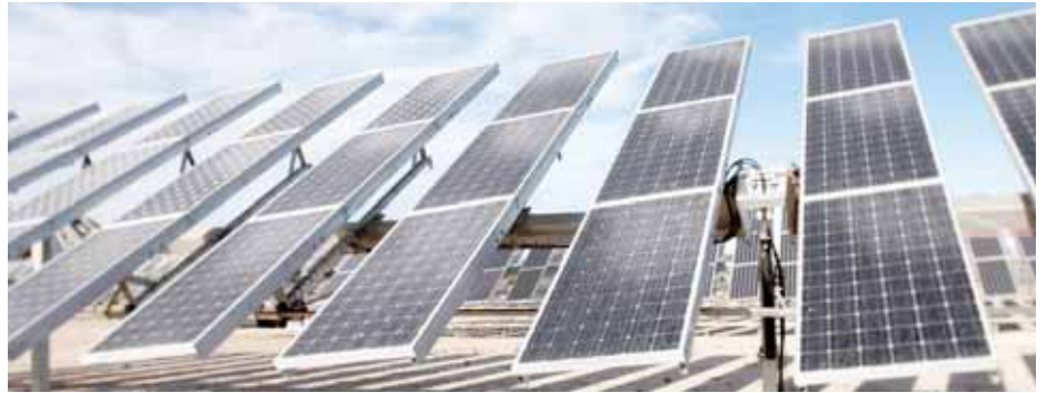
Panels at a solar power plant in Spain
