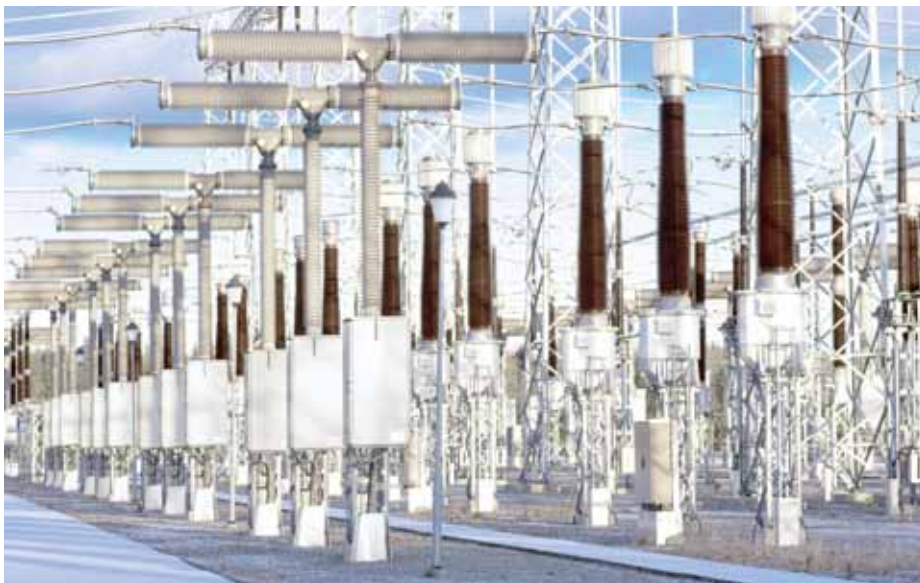
A 400 kV substation
