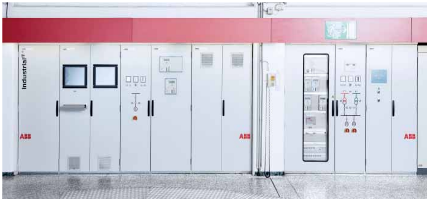
View of the control unit of a hydro power plant
