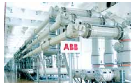
220 kV gas insulated substation
