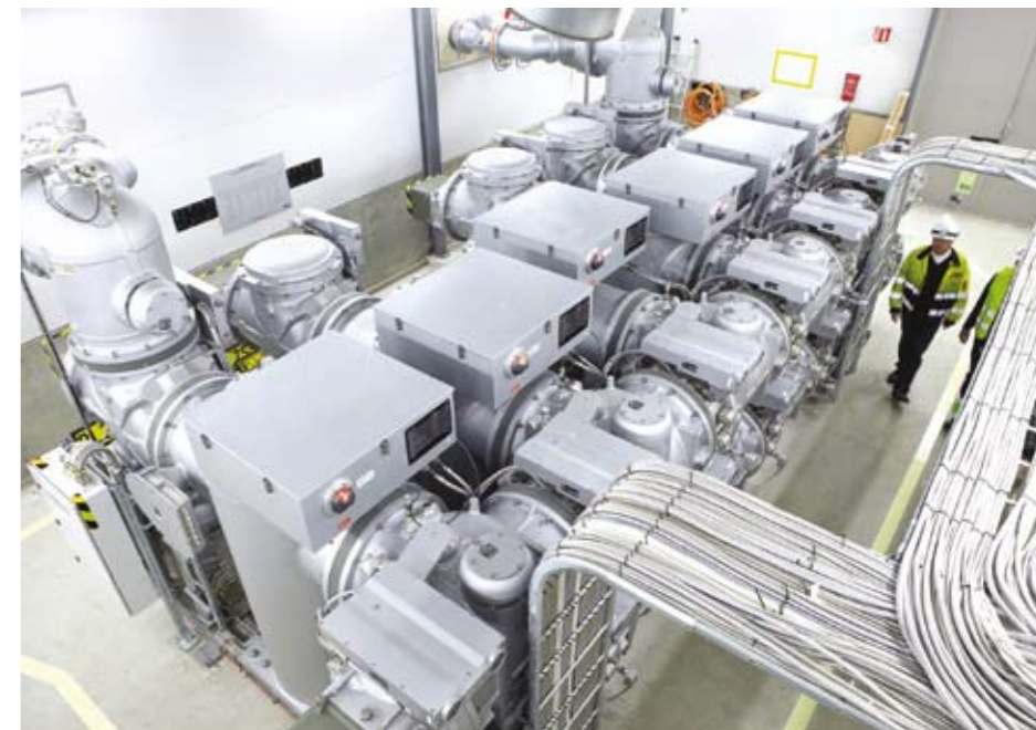
ABB – leading supplier to hydroelectric and pumped storage plants.
