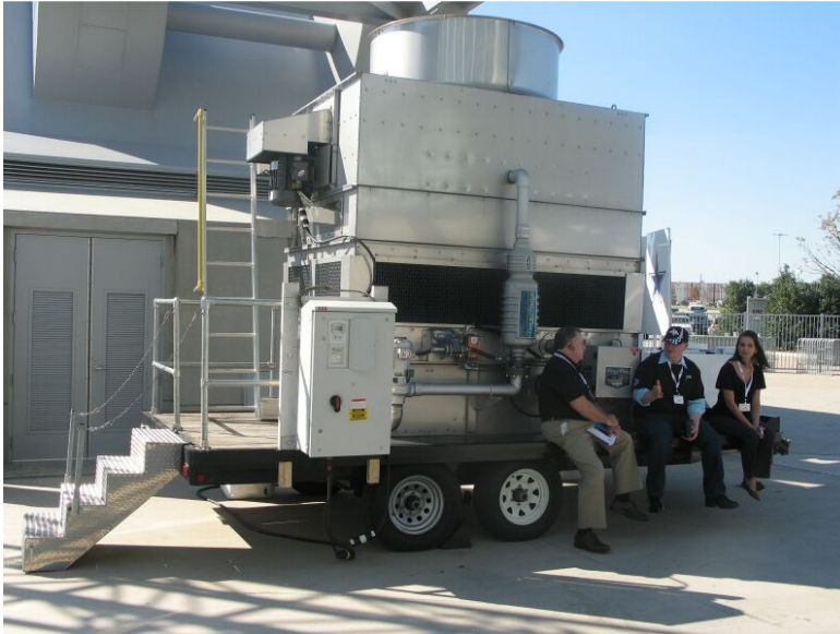
An Air Handling Unit on display outside the stadium.
