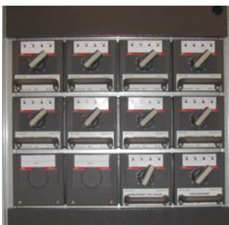
Motor control center
