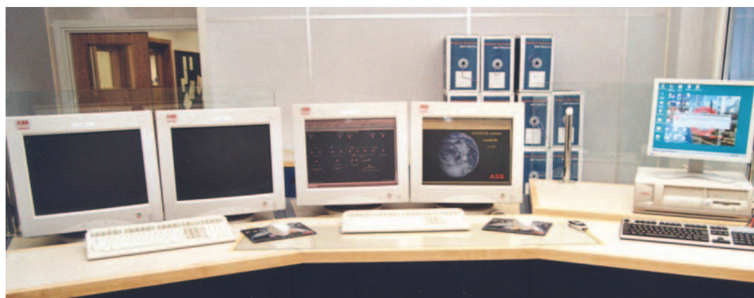
A typical control desk within the main control room from where the London Underground's power supplies system is managed.
