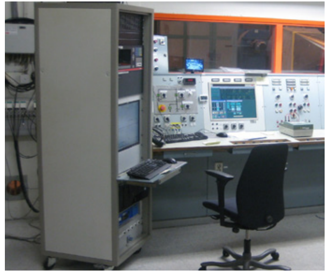
ABB Test facility
